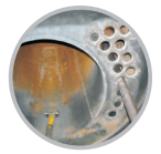
scaling in radiators
