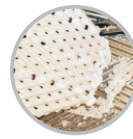
scaling in pipeline
